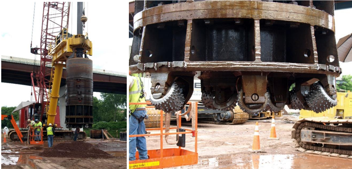
Figure 2 – Westward view of Shaft #23 construction rig near Pier 3 of job site in New Jersey (L) and close-up view of the cutterhead and cutters (R) designed for sedimentary rocks. (Dukelabs digital images taken 14 June 2013.)
