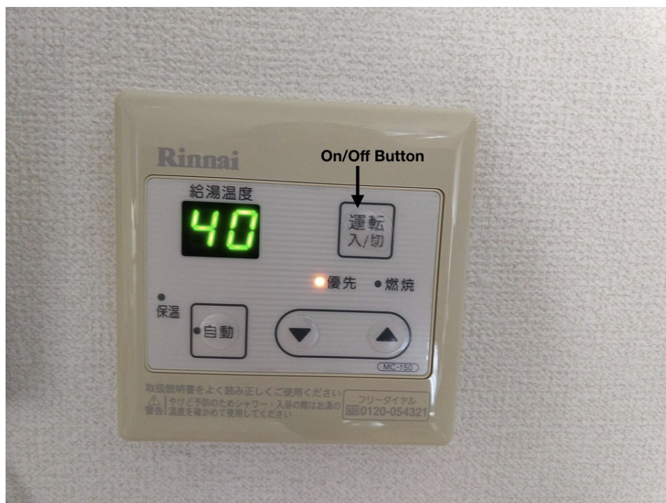
Figure 4: Hot Water Heater
